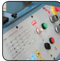
| Front Control Panel
